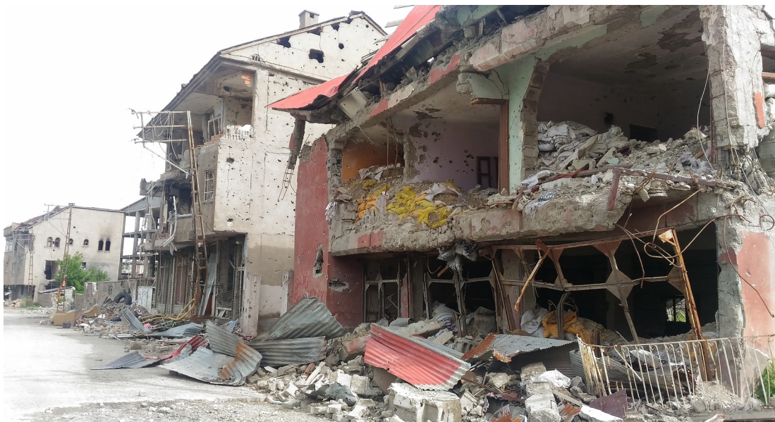
Figure 7: Destroyed building in aftermath of military operations in Yüksekova, Hakkari
